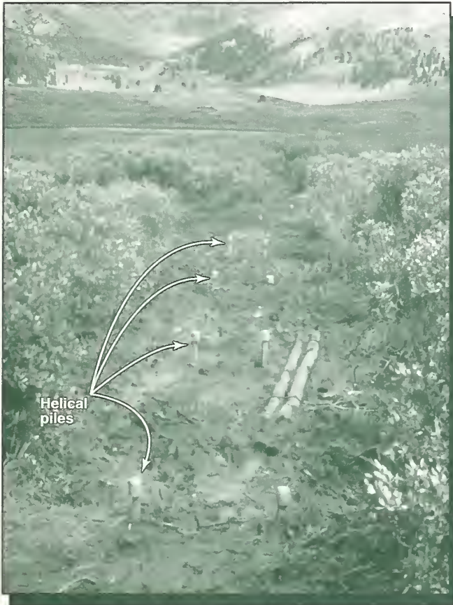
Figure 37—Helical piles installed in Colorado. The saddles are not yet attached. The ends are covered with temporary plastic caps for safety.
